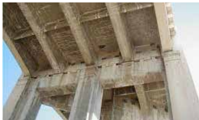
Figure 12: AAR damage in concrete
